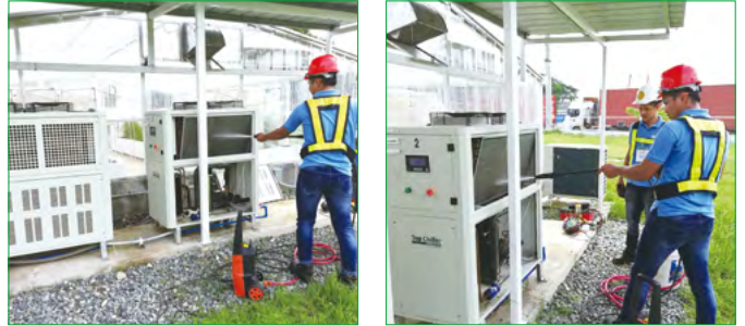
19KW 泰国风冷水机 AIR COOLED CHILLER IN THAILAND
