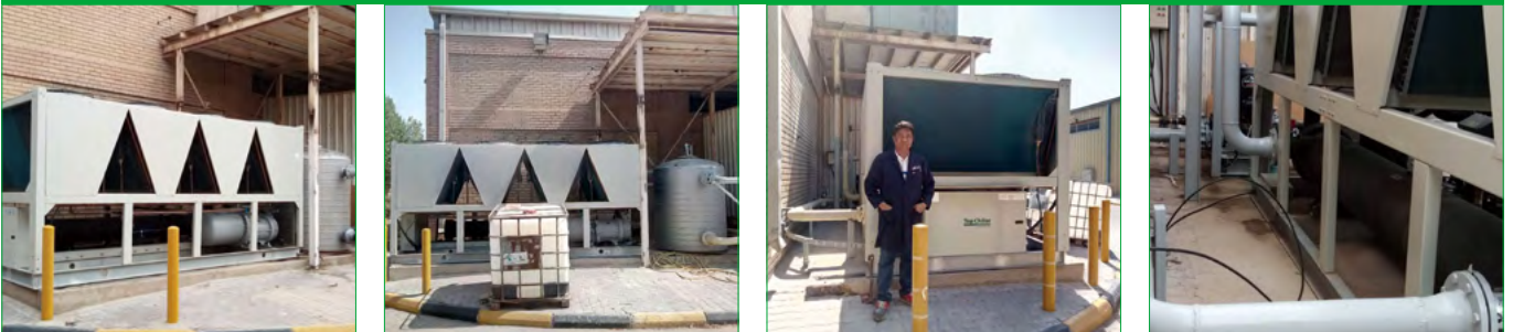
120HP 科威特风冷螺杆 AIR COOLED CHILLER IN KUWAIT
