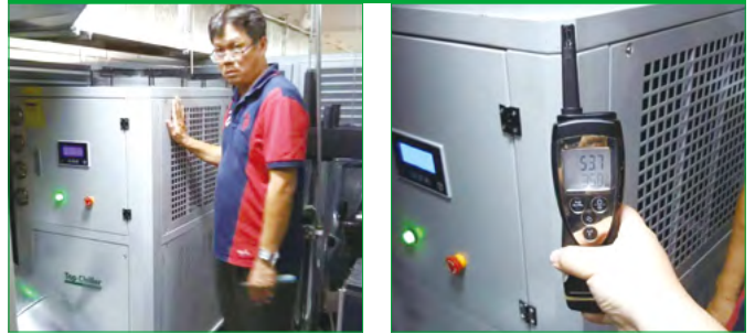
新加坡 10TON 风冷机组 AIR COOLED CHILLER IN SINGAPORE
