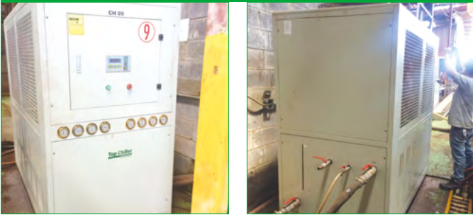
哥斯达黎加风冷 25TON AIR COOLED CHILLER IN COSTA RICA
